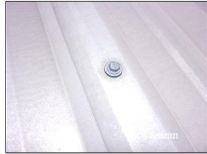
Screw In Good Condition
